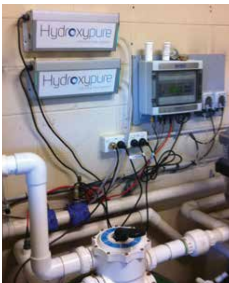
Commercial Hydroxypure system with remote access and constant monitoring.
