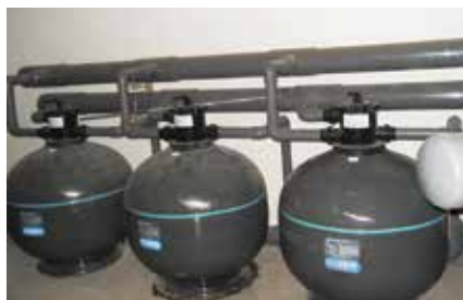
For filtration, three Micron S900 top mount fibreglass filters were installed, in addition to three Hydrostorm Plus 4HP (3-phase), variable speed pumps.
