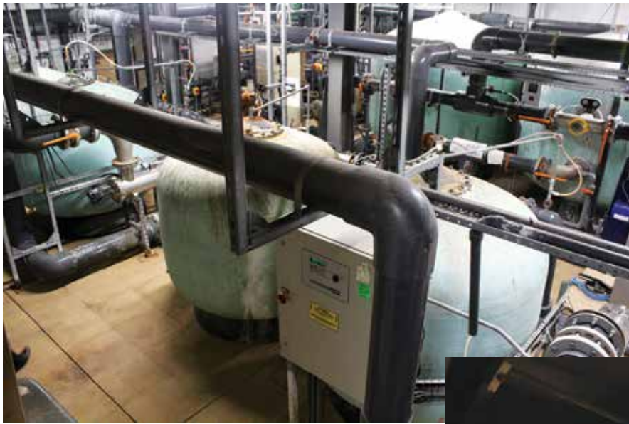
The Spa's existing filtration equipment had begun to leak and malfunction. Therefore required an immediate upgrade.
