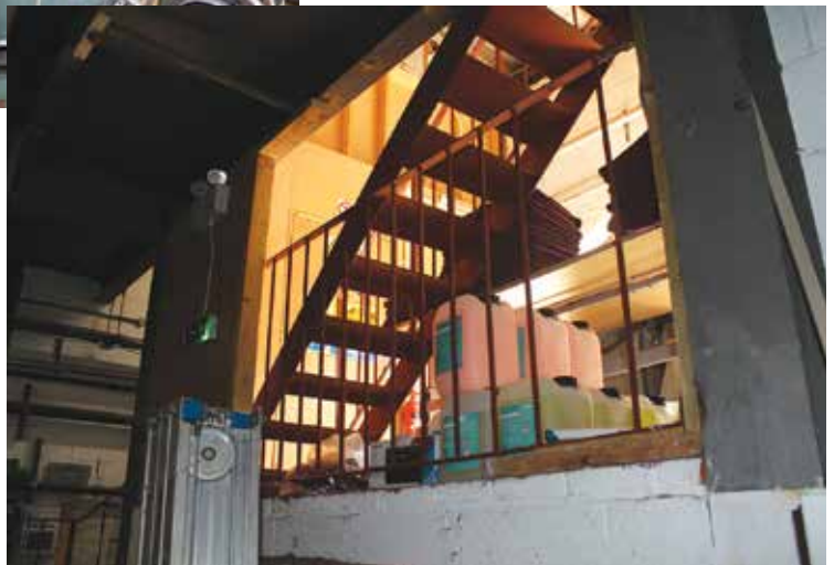
The challenge for the Nirvana maintenance team was to bring the filters in through a hole made in the wall. The problem was resolved by installing retrofit split tank filters that can be delivered in two parts and assembled on-site.
