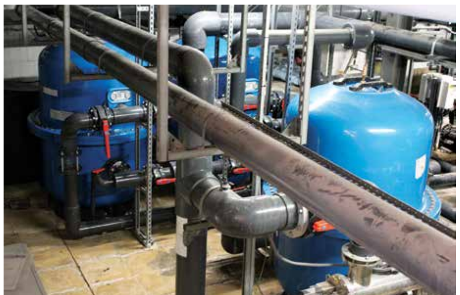
After the installation of the high quality Waterco split tanks, replacing the existing filters which had started to fail, water quality has improved for the guests and reduced backwashing for the maintenance staff.
