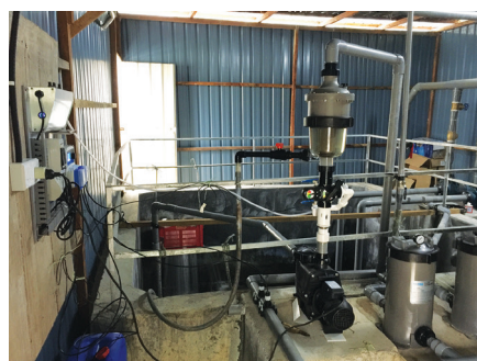
The Hydroxypure installed at the Cameron Highlands' hydroponic lettuce farm in Malaysia which is helping to improve hydroponic water quality and efficiency.
