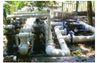
A customised Waterco MultiCyclone skid was assembled offsite and craned into Taronga Zoo.
